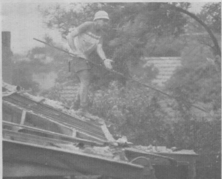
FUND RAISER —As part of a goal to raise $10,000 (Australian) for the Office Facilities Building fund, Melbourne North and West members wreck a house. Pastor Gavin Cullen (pictured) and about 75 people participated in the project, including women who stacked bricks, tile, timber and anything else that could be sold.
